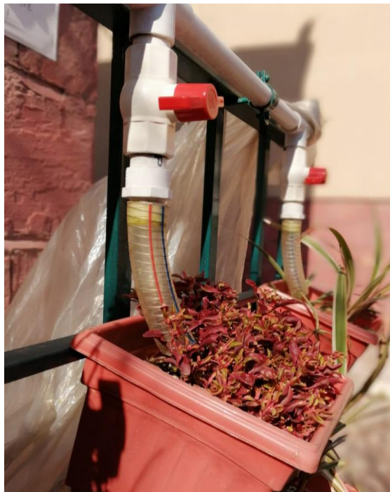
Picture 8 Flow Control Valves
