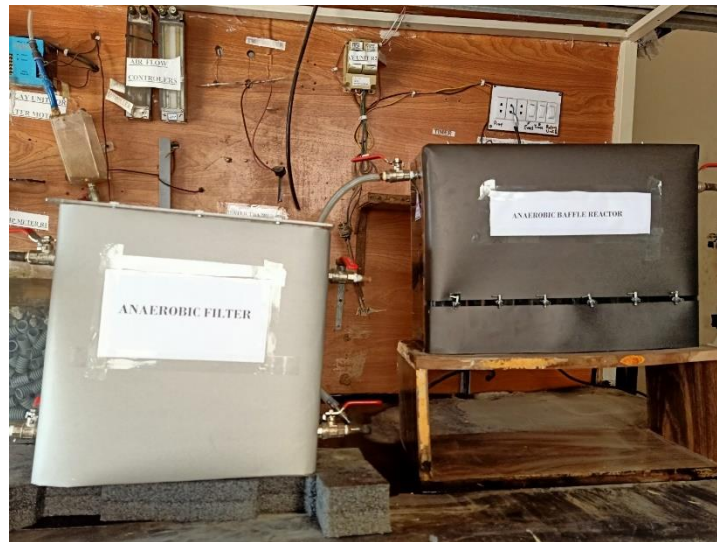
Figure 10: Covered ABR and AF Units
