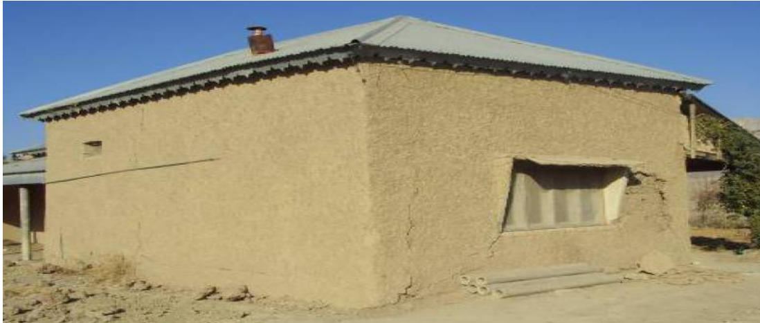
Figure 4.5: Adobe Structures or Mud Wall Structures (Structure type V), Source: field work
