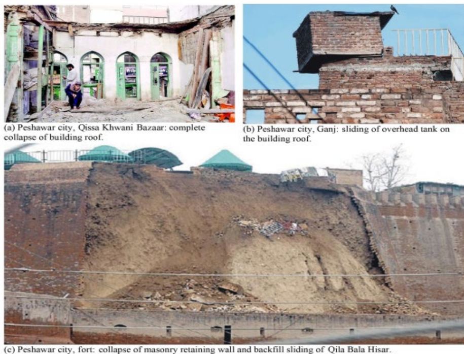
Figure 2. Damages observed in Qila bala hisar as a result of Hindukush earthquake 2015
