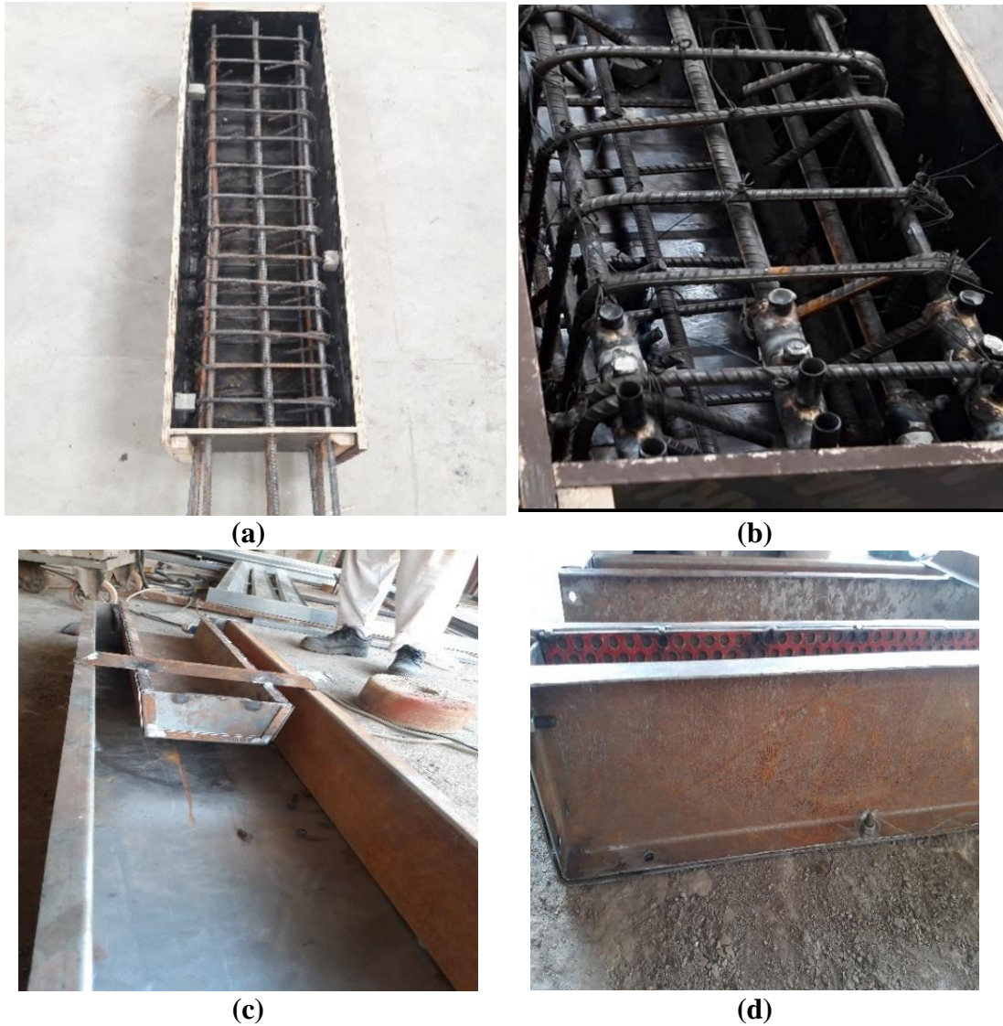
Figure 4.3. Casting of pre-cast column and formwork (a) Pre-cast lower column, (b) pre-cast upper column, (c, d) Pre-cast U shaped beam
