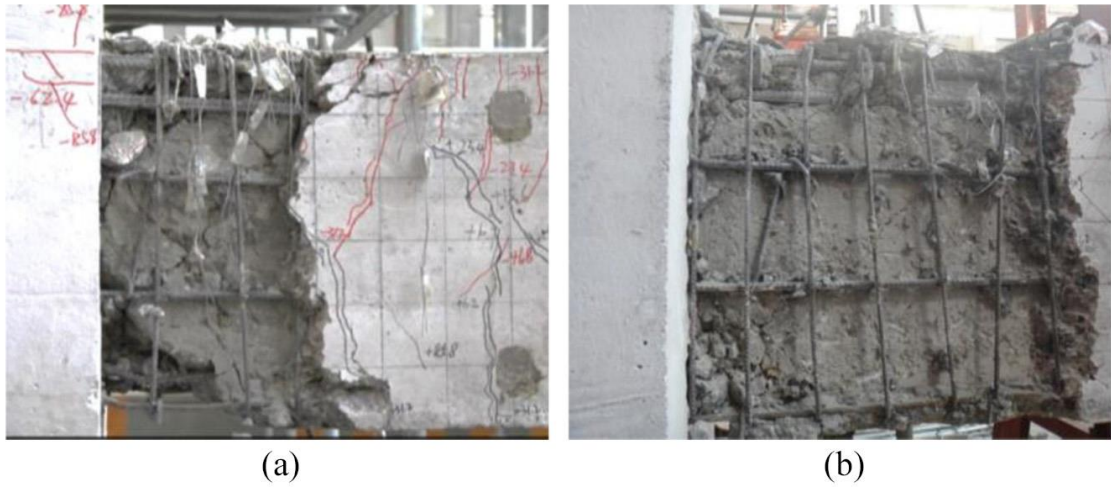
Figure 5.2. Failure modes of specimens inside the U-shaped shells: (a) SP-1 and (b) SP-4.
