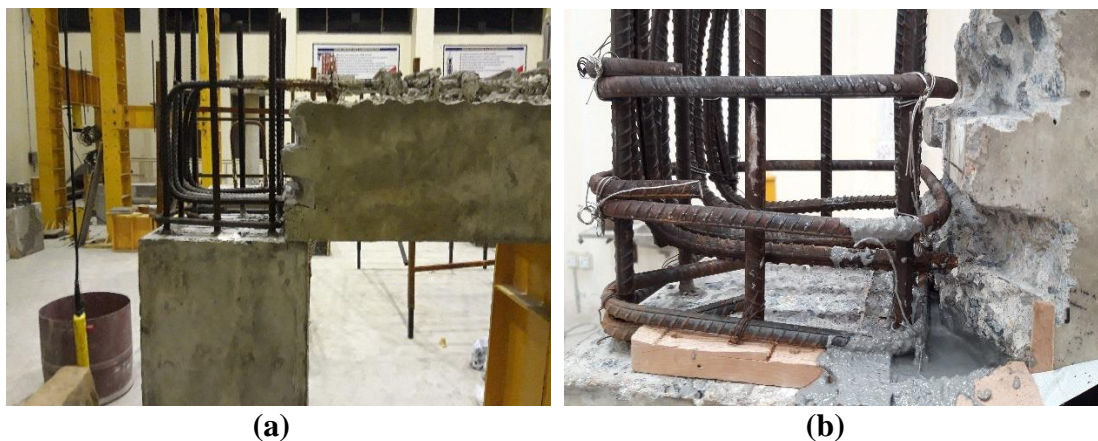
Figure 4.4. Shows the Assembling of pre-cast beam on joint (a) Placement of U-beam on column, (b) Joint region of beam-column joint under consideration.
