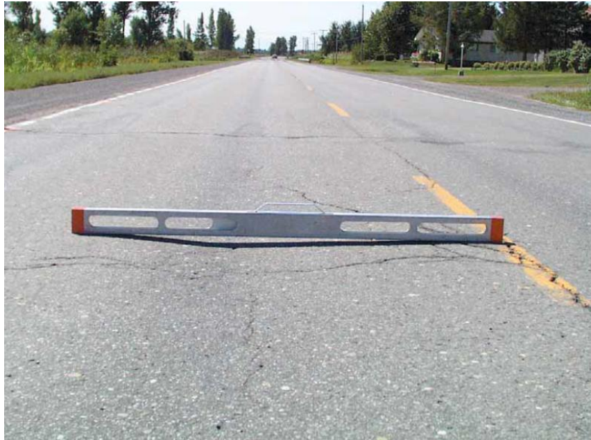
Figure 3.11 Rutting in Asphalt Pavement
