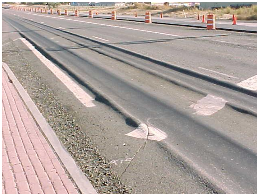
Figure 3.12 Severe Mix Rutting in Asphalt
