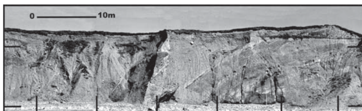
Figure 6.27 Dinas Dinlle photo mosaic constructed from six overlapping digital images with 10m markers overlain. This mosaic can be used to construct a technically accurate sketch of the outcrop.
