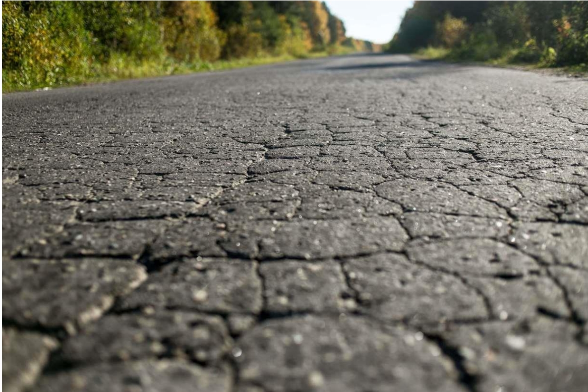
Figure 1.2 (b) Cracks can be seen on a flexible pavement.
