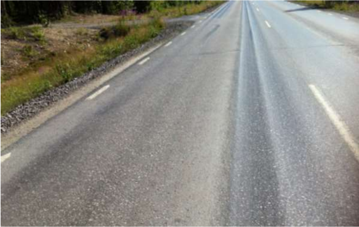
Figure 2.1: Rutting Defect in Flexible Pavement ( https://www.roadex.org )
