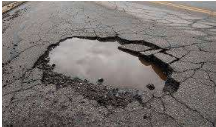
Figure 2.2: Observed Water damage of Flexible Pavement
