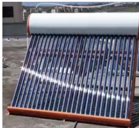
Figure 19: Solar water heater
