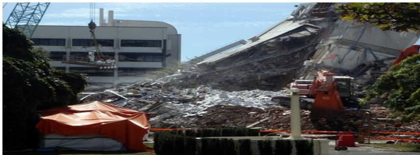
Figure 1.1: The collapsed building of PGC [14]
