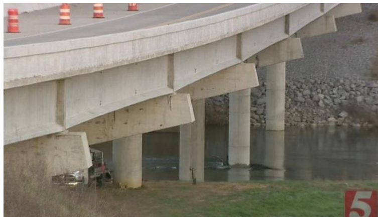
Figure 1.1– Structural Damage in a bridge
