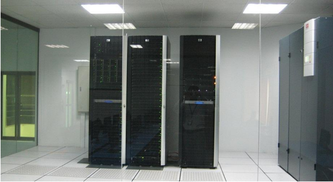
Figure 4.1: Physical Data Center at RCMS, NUST
