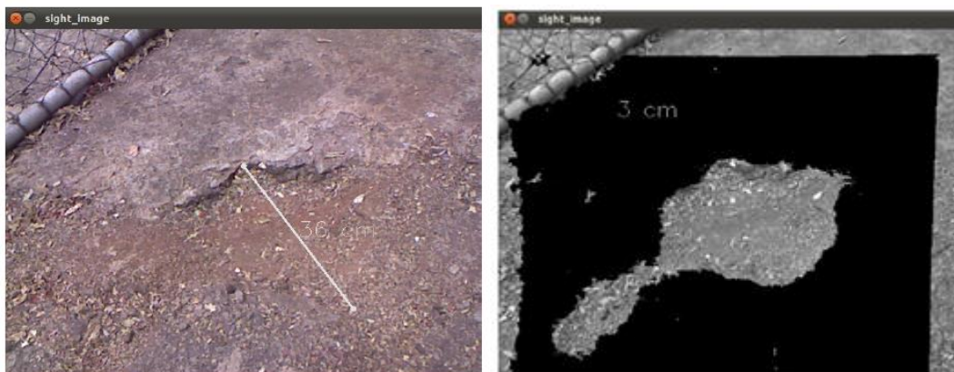
FIGURE 2.17. POTHOLE MANUAL WIDTH AND DEPTH MEASUREMENT [21]
