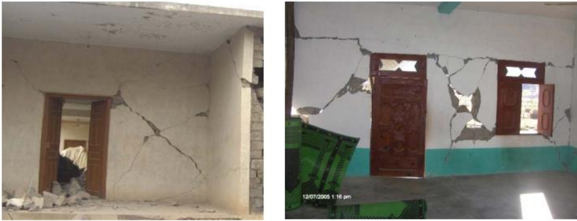
Figure 1- 2: In plane failure of masonry building
