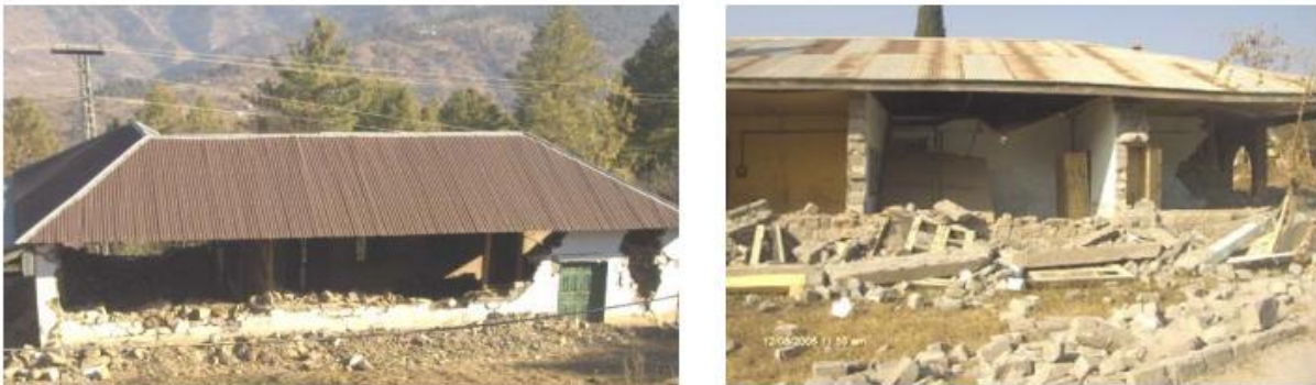
Figure 1- 3: Out of plane bending failure of masonry walls
