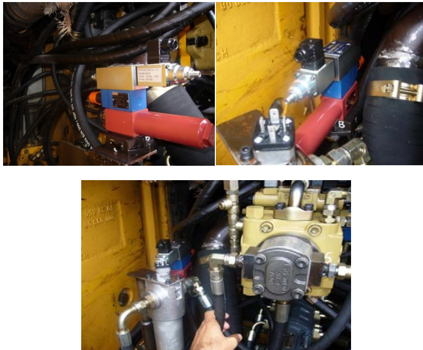
Fig 6.3: Valves installed in the crane LIEBHERR HS885HD with the pump.
