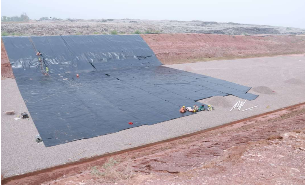
Figure 2 On-going Construction of Sanitary Landfill at Shamshatoo, Peshawar (Source: WSSP LinkedIn Profile)
