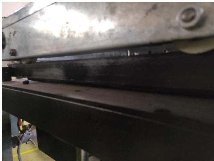
Figure 25. Heater's wheels travelling on the heater rails
