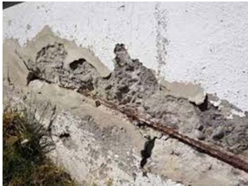
Figure 4-4- Conventional Steel Formwork, Steel Cover Problem
