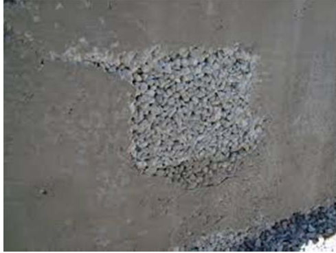
Figure 4-3- Conventional Steel Formwork, Honey Comb Problem
