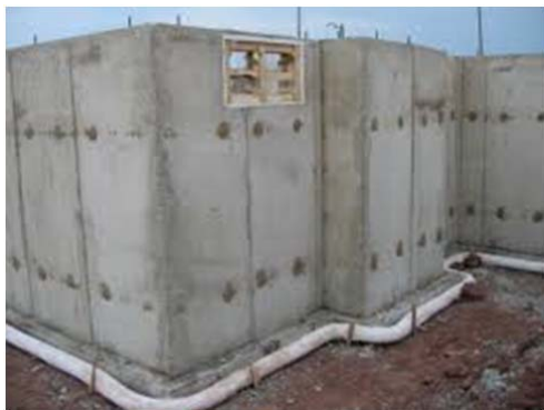
Figure 4-5- Conventional Steel Formwork, Verticality Problem
