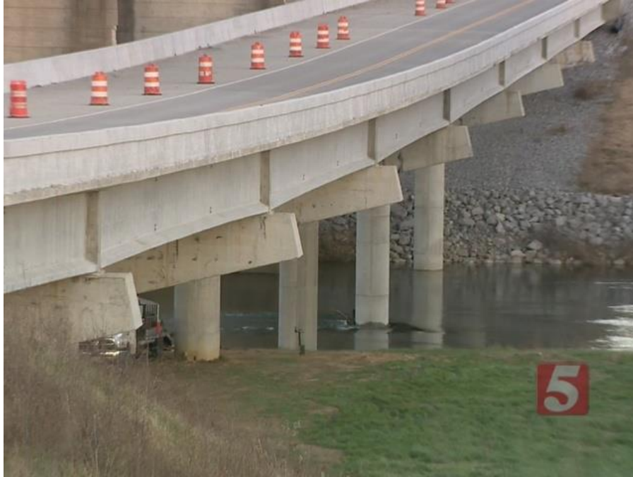
Figure 1-1: Structural damage in a bridge
