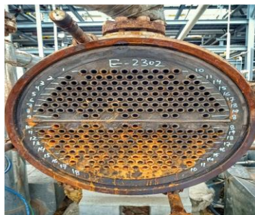
Figure 20. Inspection of tube through RFT and numbering of tubes
