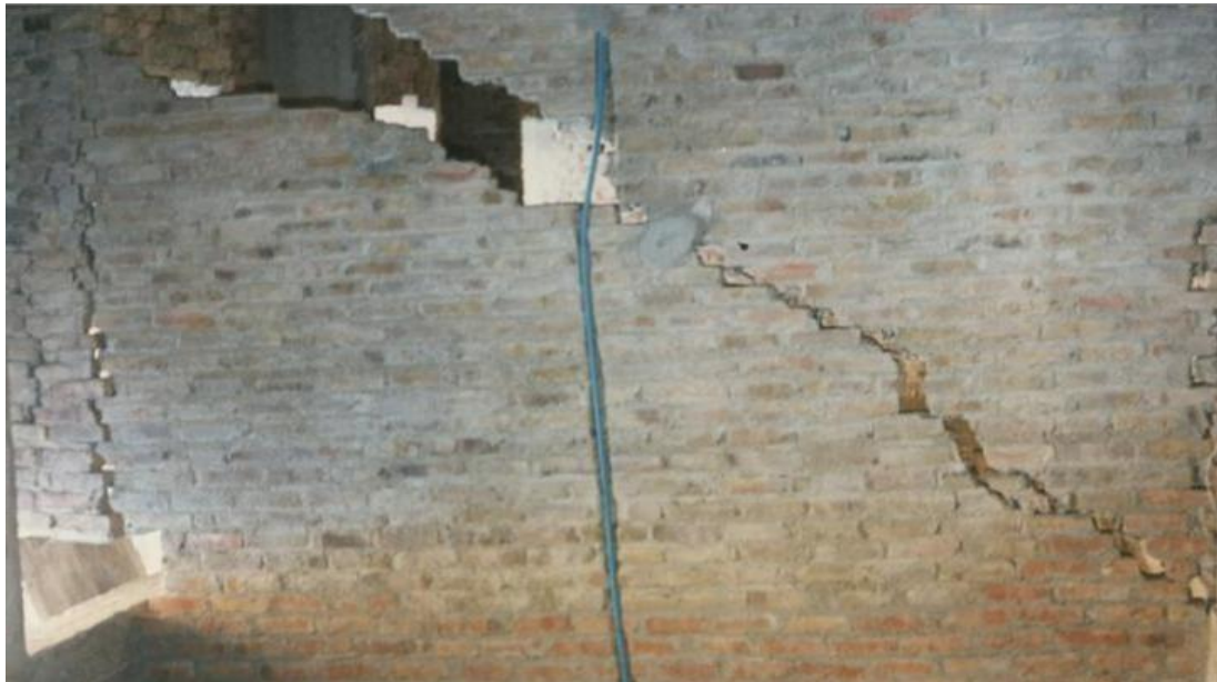
Fig 2.7 Crack in wall due to the Uplift pressure of the clay.
