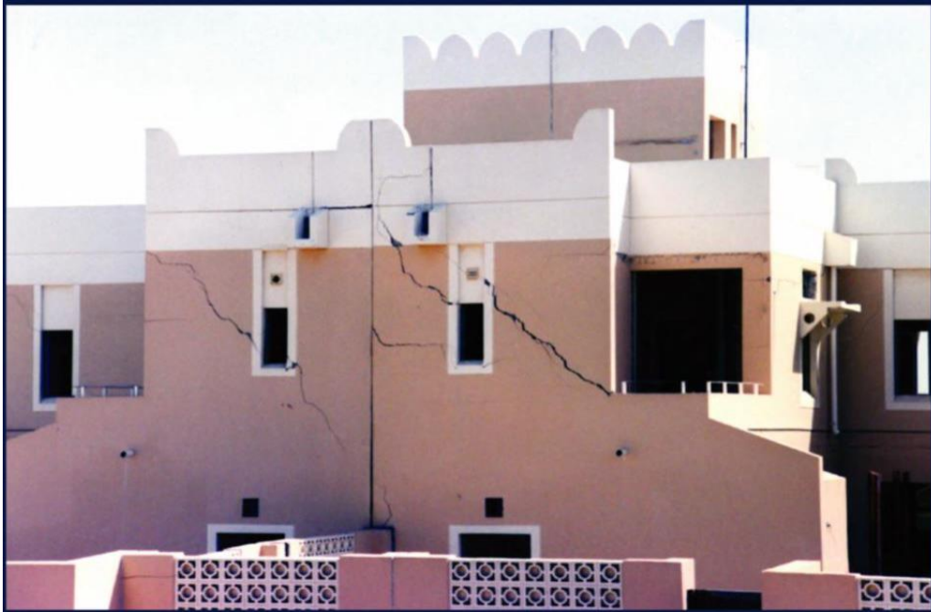
Figure 2.2 Cracks in walls of residential buildings
