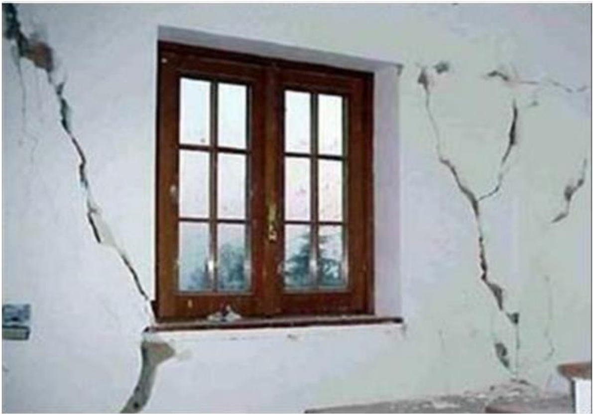
Figure 2.4 Cracks in walls of single storey building
