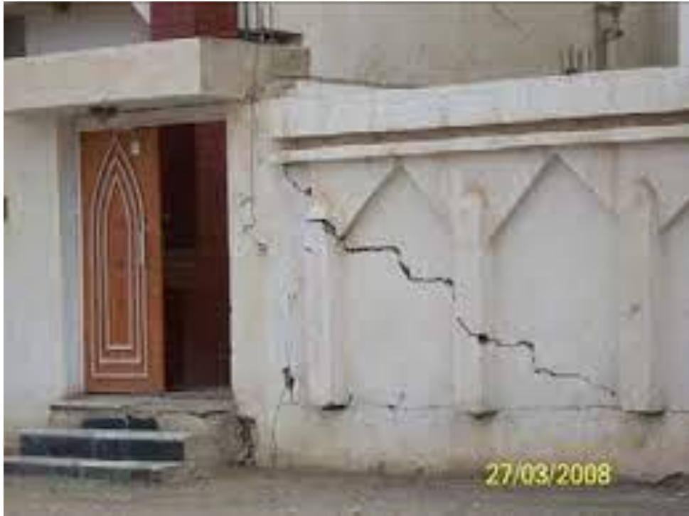
Fig 2.6 Crack in boundary wall due to the Swelling clay.
