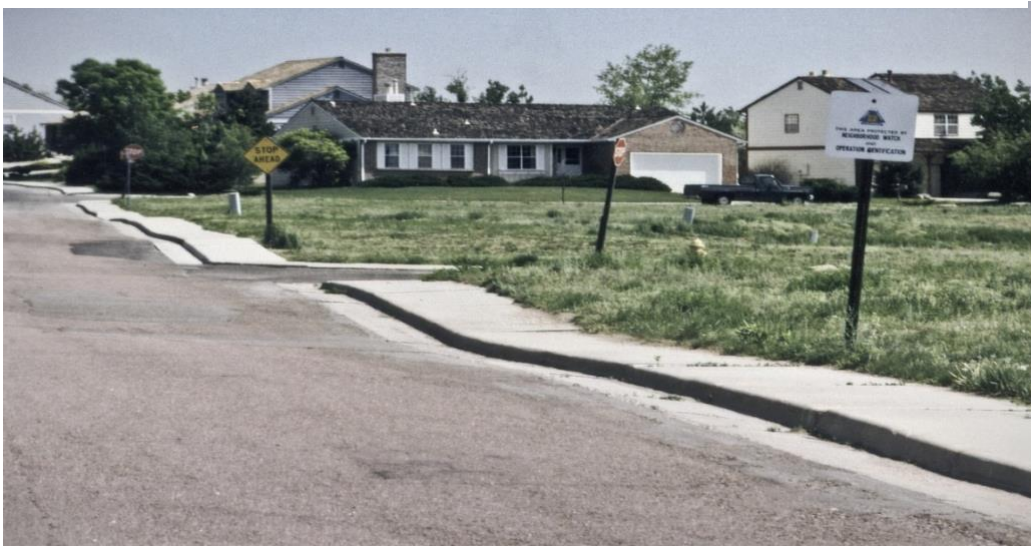
Figure 2.3 Damage to a flexible pavement due to swelling of clay
