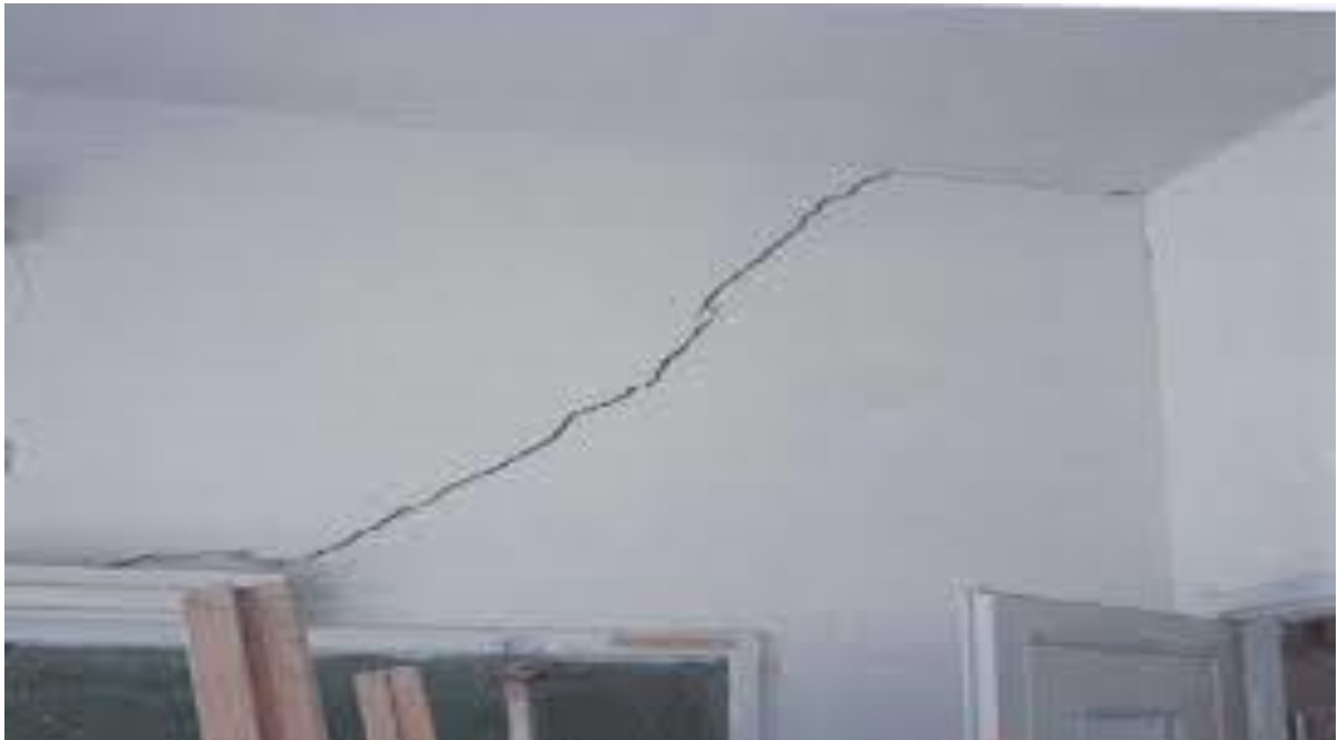
Figure 2.5 45 degree crack in a wall due to uplift pressure
