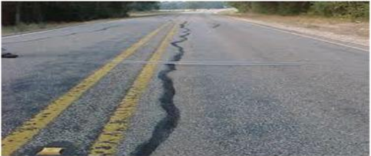
Fig 2.1 Damage to road due to the uplifting of underneath expansive soil
