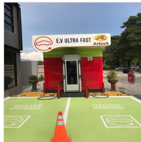
Figure 8. EV Charger Installed at APL Blue Area Site
