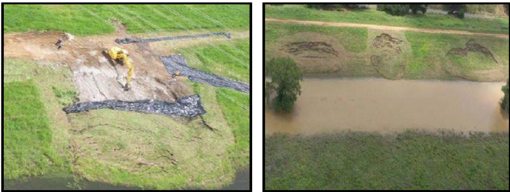
Figure 2.1: Shallow slope failures
