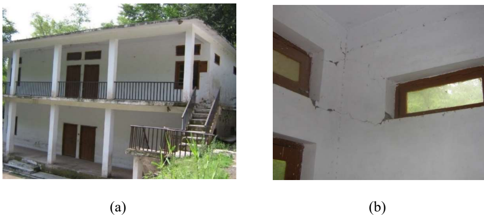
Figure 3.6: Diagonal adjoining cracks due to stress concentration near openings: (a) isometric view of school; (b) Shear cracking due to stress concentration near openings
