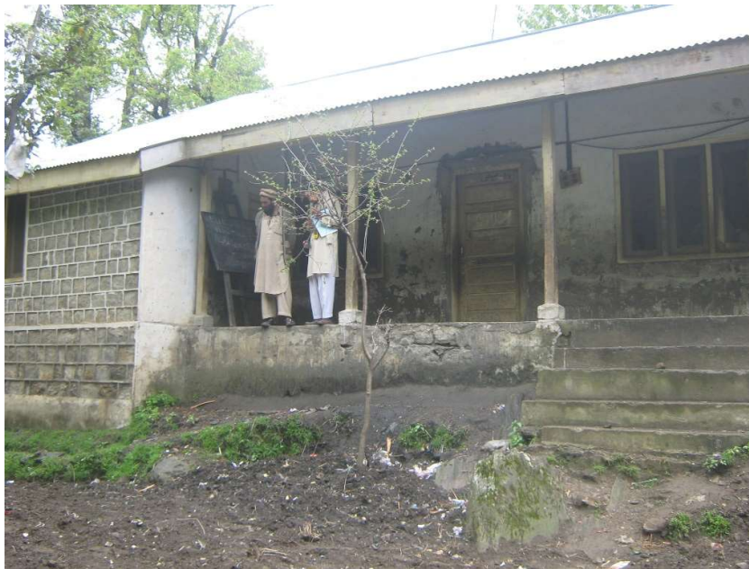
Figure 4.27: A photograph of typical stone masonry block, showing the adjoining toilet, repaired door, and flexible diaphragm
