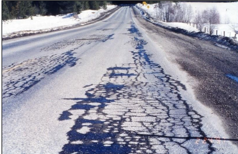
Figure 2.2: Soil frost action caused damage to the pavement
