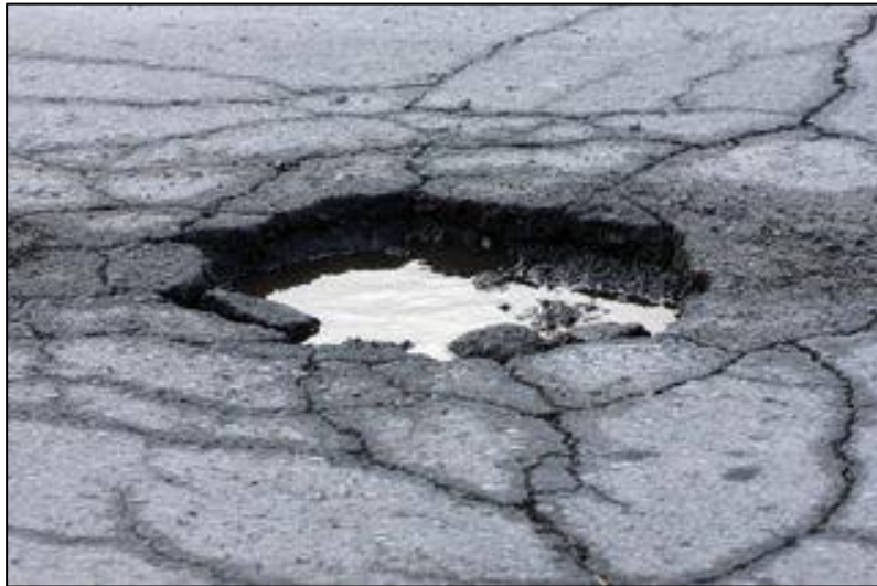
Figure 2.3: Pothole formation due to subgrade erosion
