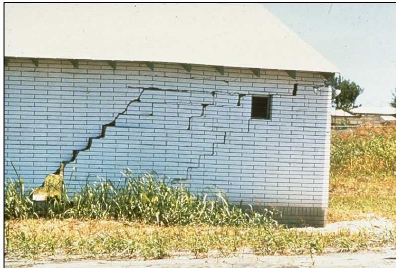
Figure 2.1: Cracks in building walls due to clay shrinking
