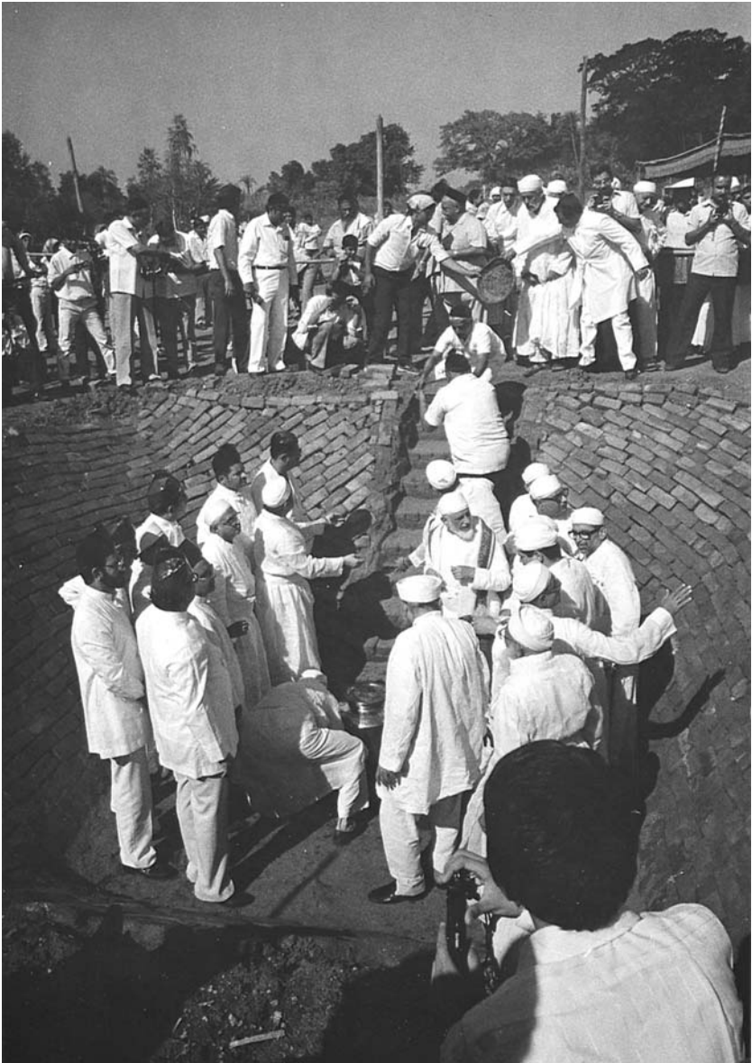
6. Installation of the foundation for a new fire temple at the site of the first Parsi landing in Gujarat. Courtesy of Professor T. M. Luhrmann.
