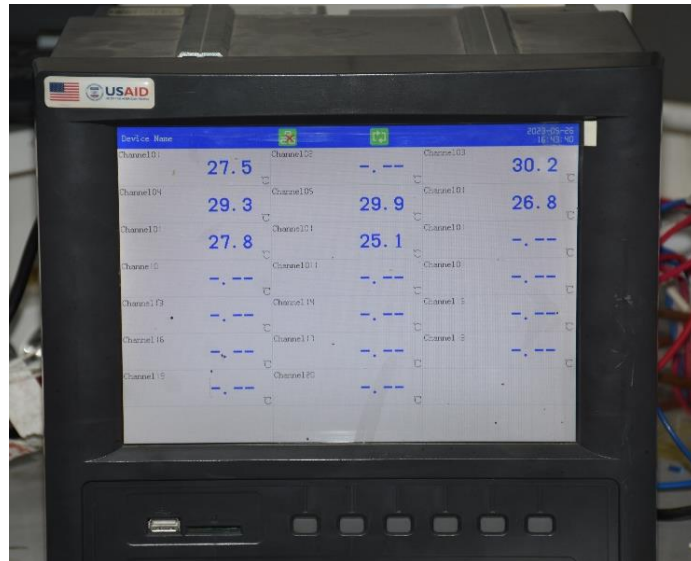
Figure 3.4. Temperature data logger
