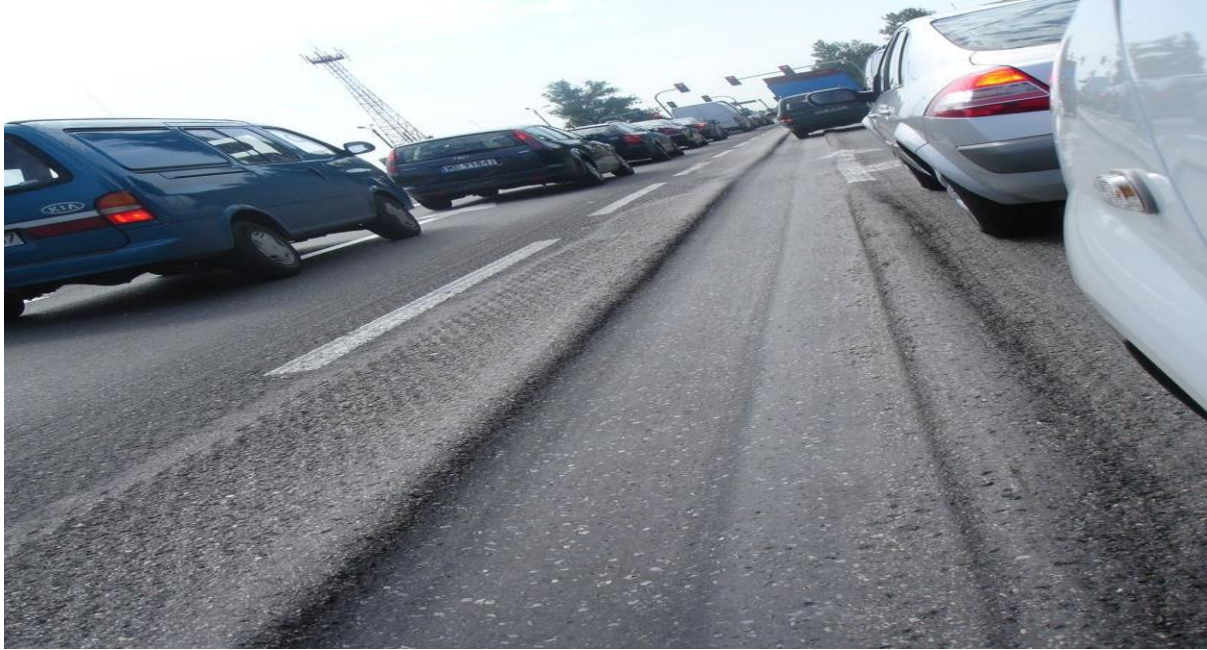
Figure 2.3 Rutting in Pavement
