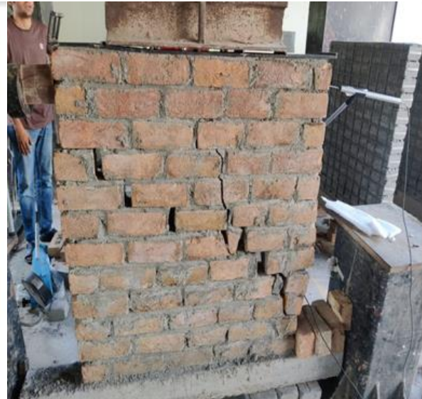
Fig 4.2: Stepped Cracking of Wallet
