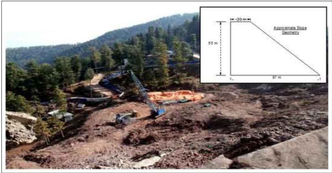
Figure 2 Jhika Gali Landslide [8]
