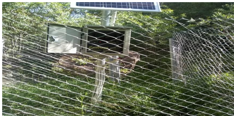
Figure 5.2 Water Station operating Equipment's
