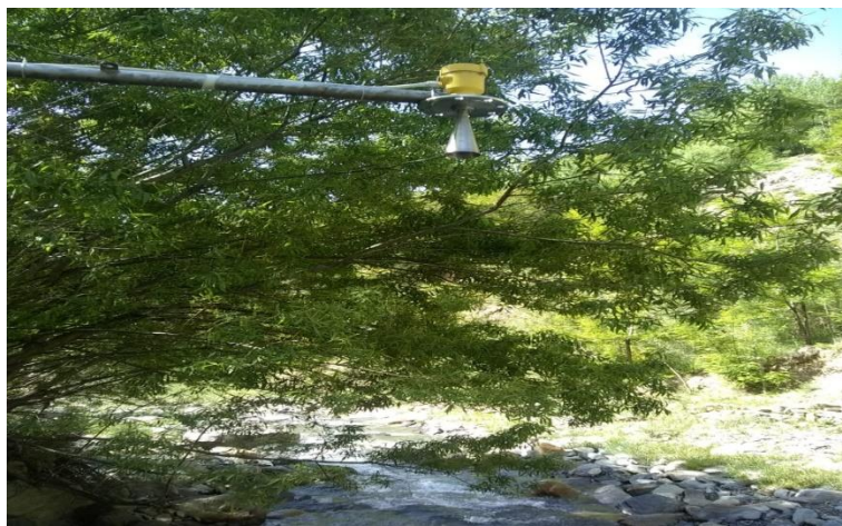
Figure 5.1 Installed Radar Sensor
