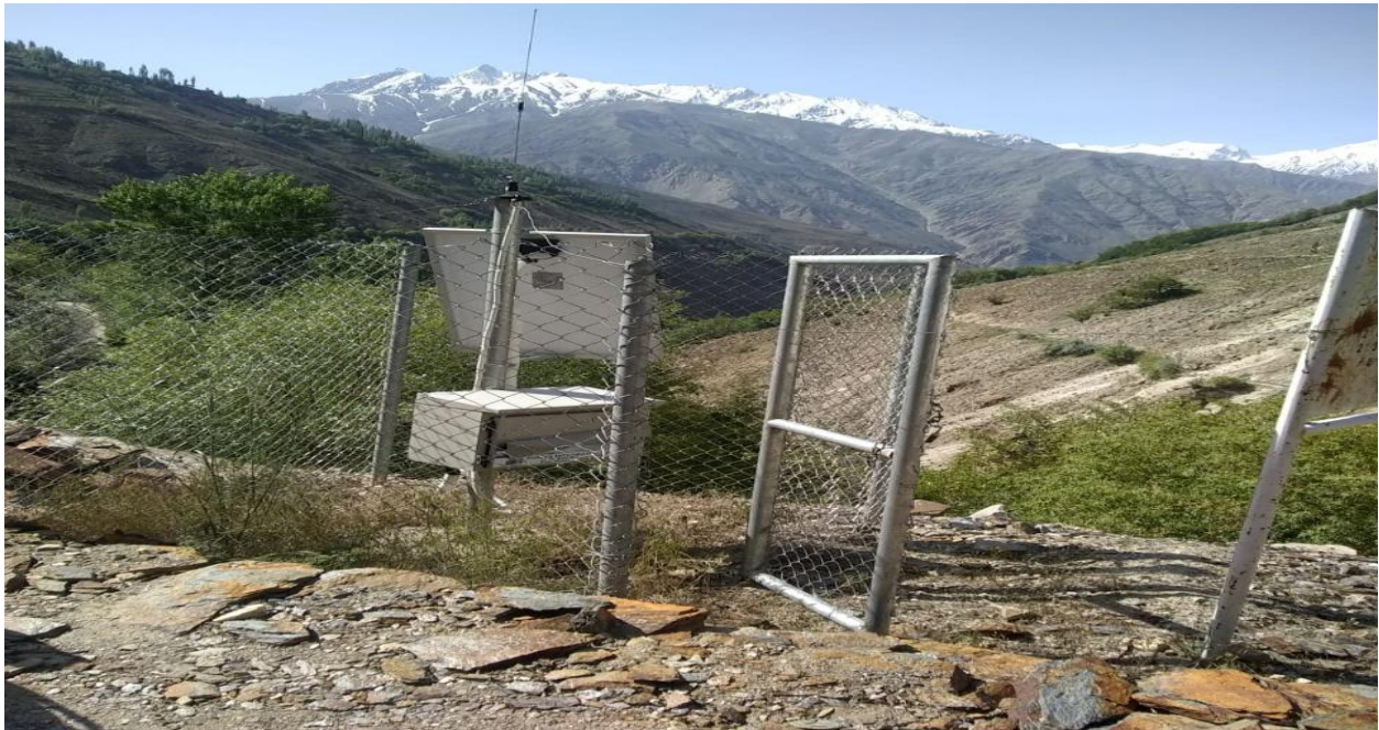
Figure 5.3 Repeater Station Operating Equipment's
