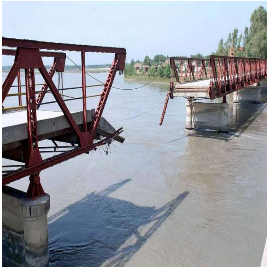
Figure 1.1: Sardaryab Bridge Collapse.
