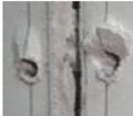
Figure 1.15: Pull through failure [9]
