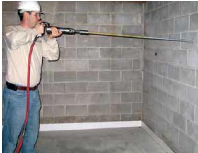
Figure 2.3 Drilling hole inside wall for tie rod installation (Helical Piles and Anchors Hydraulically Driven Push Piers Polyurethane Injection Supplemental Support Systems, n.d.)
