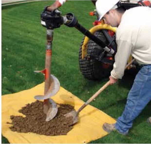
Figure 2.2 Drilling hole in soil for vertical plate anchor installation (Helical Piles and Anchors Hydraulically Driven Push Piers Polyurethane Injection Supplemental Support Systems, n.d.)
