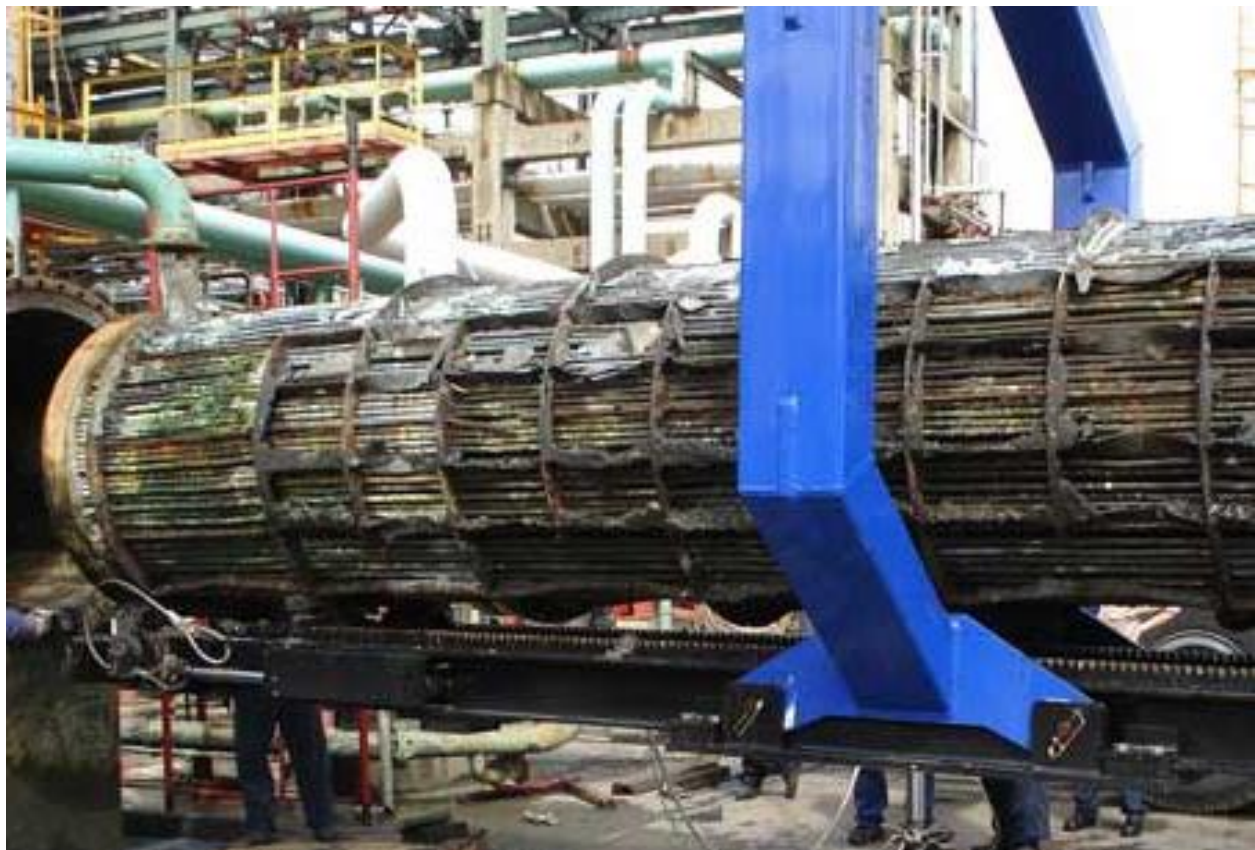
Figure 7: Disassembly for Heat Exchanger Maintenance. *
