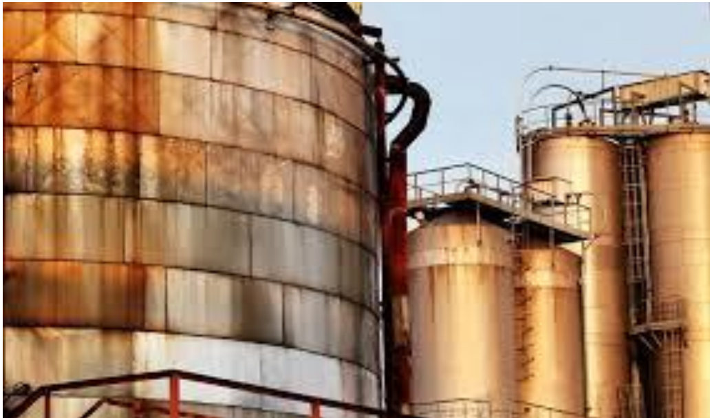
Figure 1.1: Atmospheric corrosion effects in industrial sector [9]
