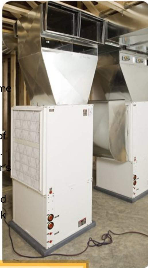
This machine is part of a geothermal heat pump system. The machine pumps the water.
