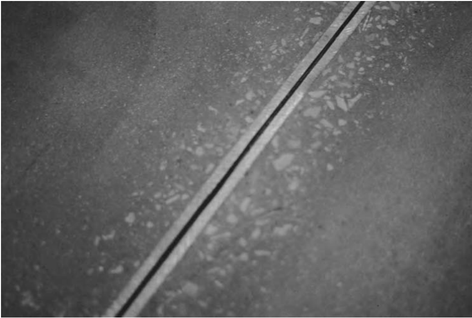
Figure 15.8 This armoured joint (flat-bar type) needed grinding
