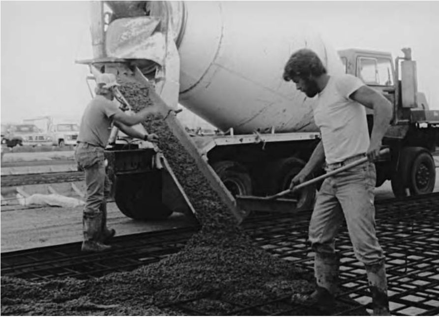
Figure 7.1 A slump of about 100–125 mm (4–5 in), as shown here, often works well in slab construction
