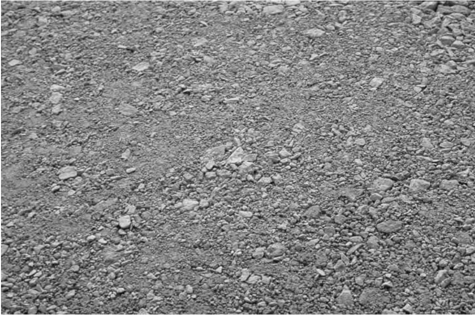
Figure 5.2 All-in crushed rock, with a blend of coarse and fine particles, makes a good sub-base
