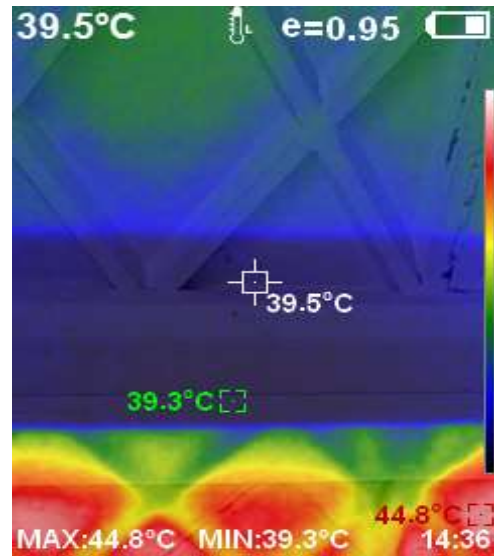
Figure 20. This picture was taken at the ceiling at 02:36 PM on Day 02. It is clearly seen that the temperature of ceiling whose roof is not covered with wet terracotta tiles is at 44.8°C and the ceiling covered with wet terracotta tiles is at 39.5°C
