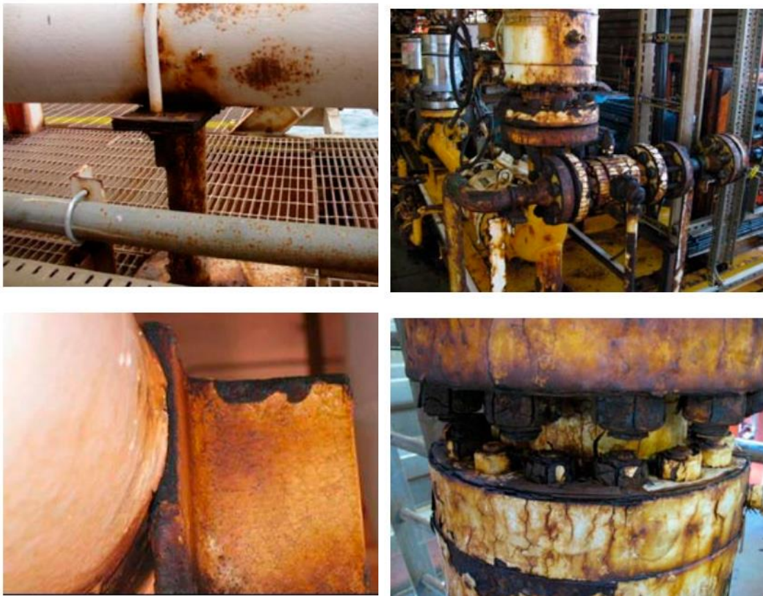
Figure -1: Example of corrosion effects on bolts, valves and pipes [2]
