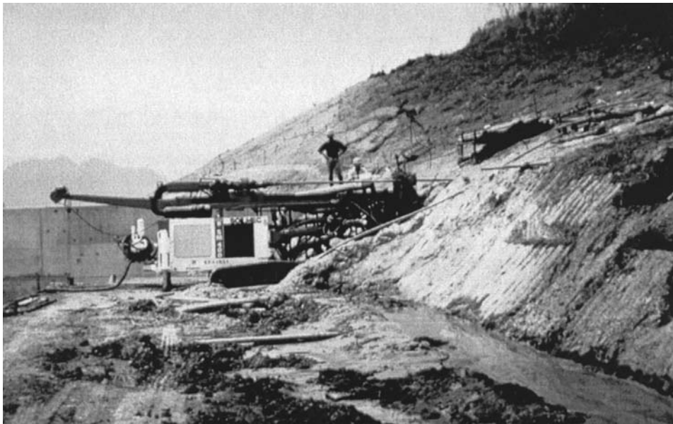
Figure 16.2 Drilling horizontal drains in the right abutment of La Esperanza Dam in Ecuador.
