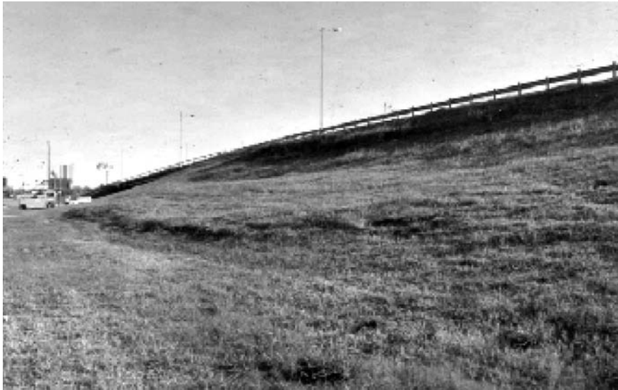
Figure 2.5 Slide in highway embankment near Houston, Texas. Embankment constructed of highly plastic clay.
