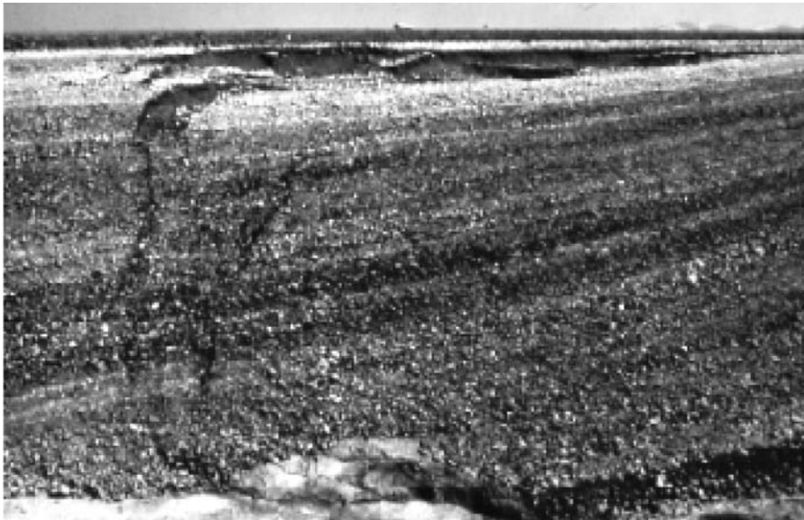
Figure 2.6 San Luis Dam upstream slope failure.
