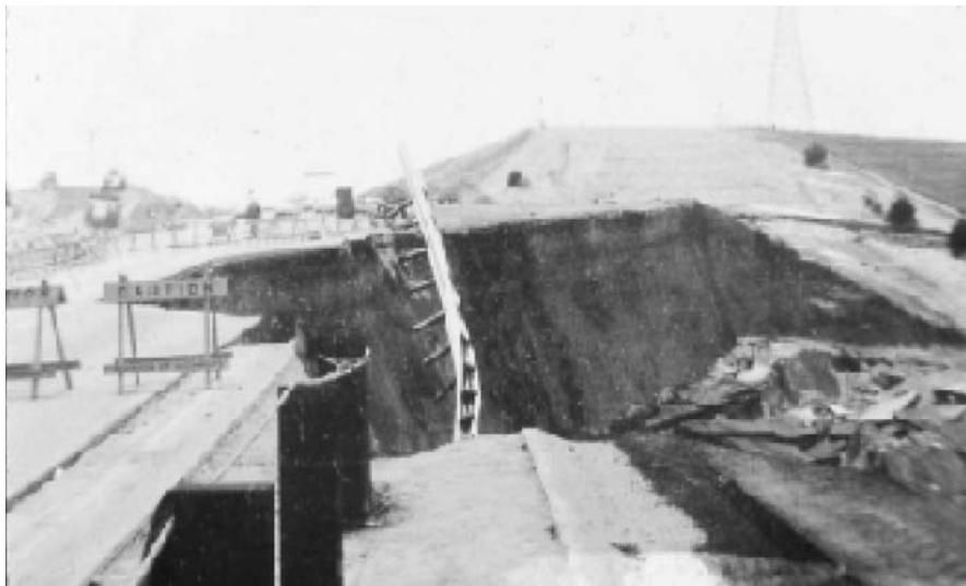
Figure 2.4 Interstate 80 embankment slope failure.
