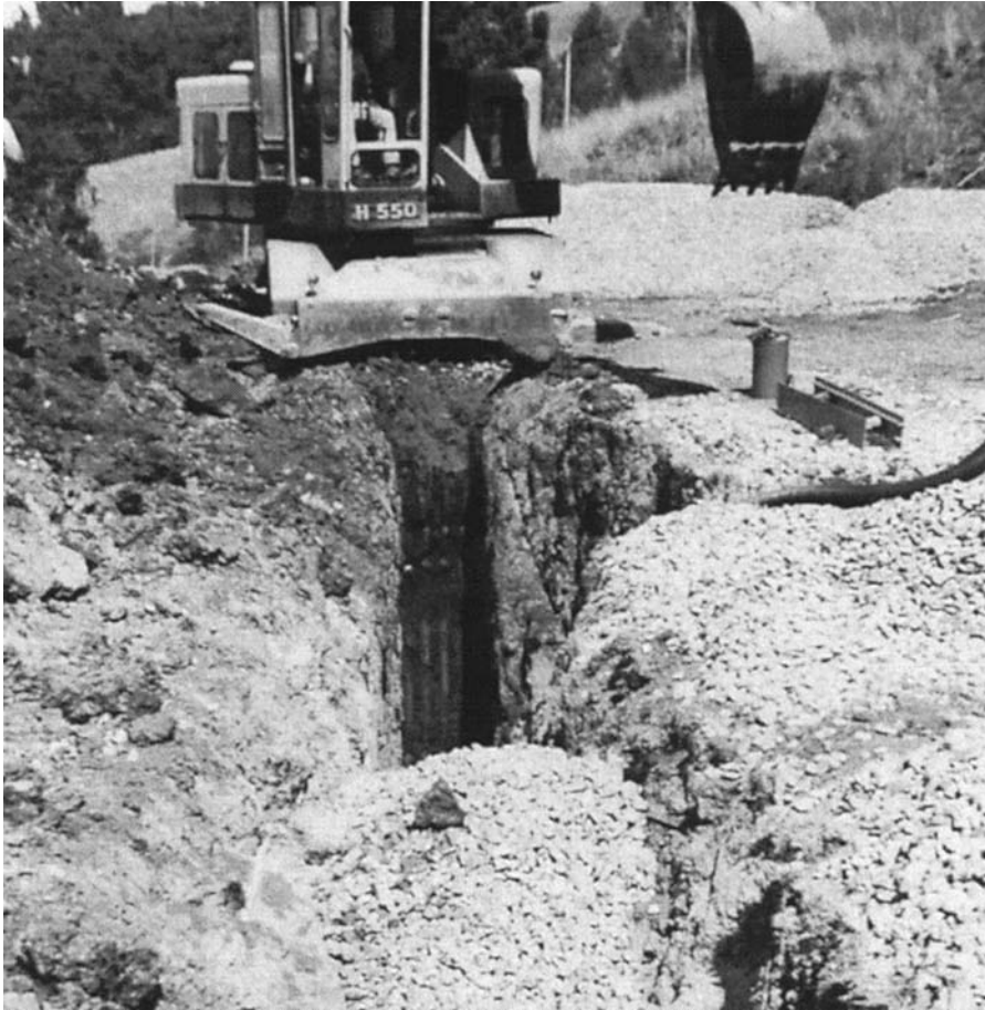
Figure 16.7 Trench drain at Lawrence Berkeley Laboratory.
