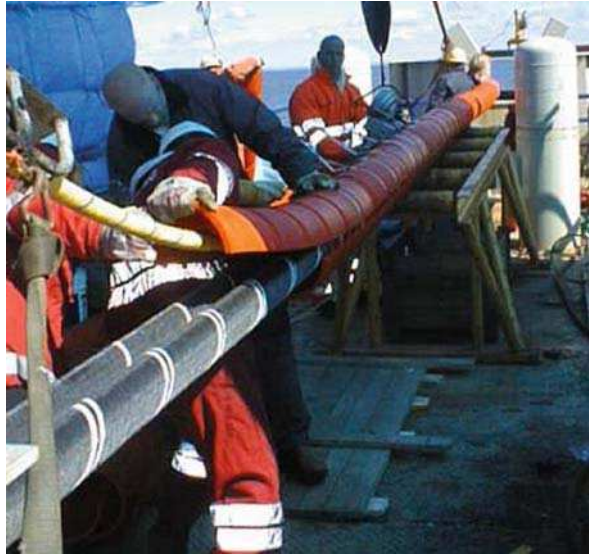
Fig. 7.23 Protective plastic shells are attached to two HVDC cables and an FO cable before the cable group leaves the vessel (Courtesy of ABB, Sweden)
