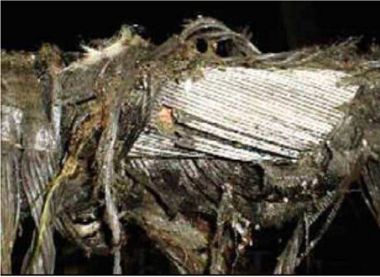
Fig. 8.3 Anchor damages on the 120 mm Baltic Cable (Courtesy of Baltic Cable AB, Sweden) [7]
