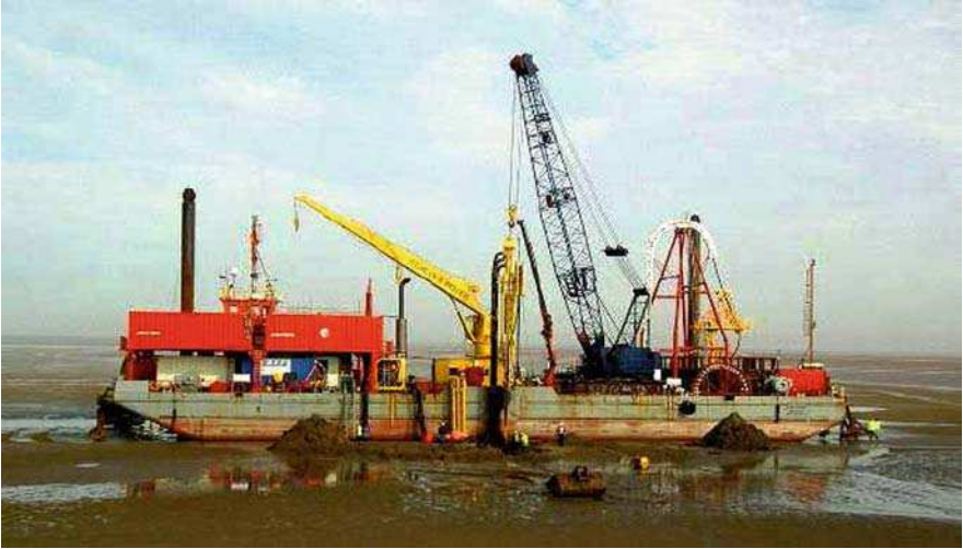
Fig. 7.3 Flat bottom barge mobilised for cable laying in tidal flats (Courtesy of Oceanteam Power and Umbilicals, UK)
