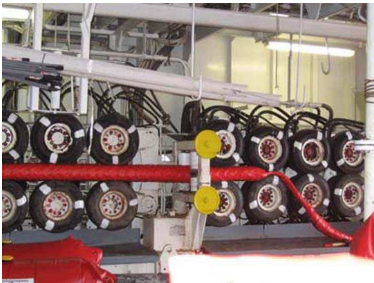
Fig. 7.9 Cable tensioner with eight wheel pairs taking grip of the leading cable end
