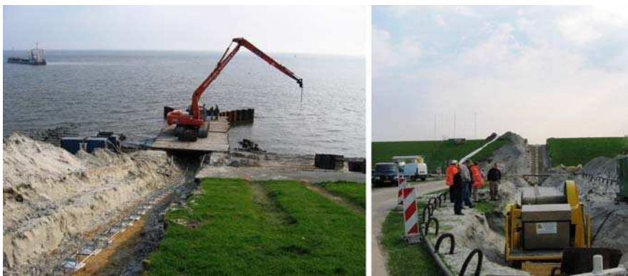
Fig. 7.14 Landing of a submarine power cable (NorNed) in open trench over the protection wall. In the splash zone, an open pit was created with cofferdam walls to receive the cable. The cut in the dike is visible in the distance in the right picture. Cable winch is in the foreground
