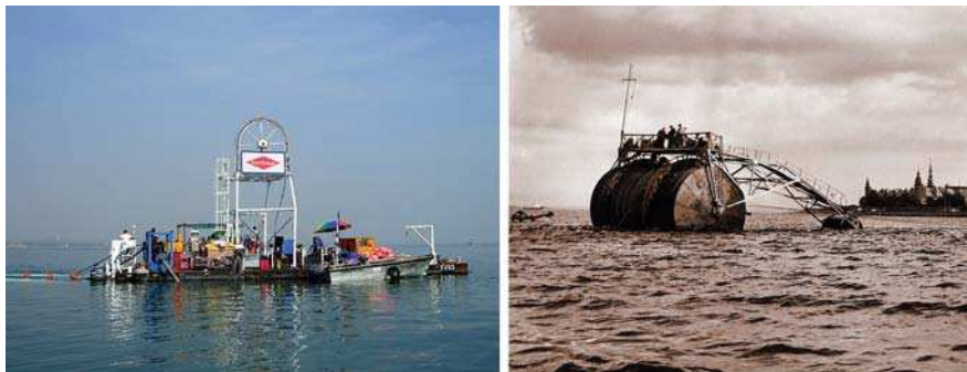
Fig. 11.3 (a) Purpose-built cable laying arrangement for calm waters. (b) Floating cable drum used as laying vessel. (Courtesy of NKT Cables A/S)
