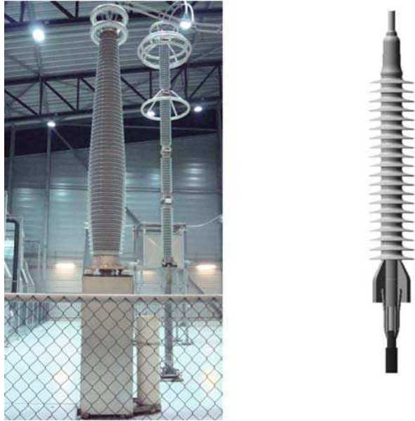
Fig. 4.8 Indoor HVDC cable terminations for mass-impregnated cable ( left ) and extruded cable ( right ). Small oil reservoir cylinder is attached to the stand of the left termination
