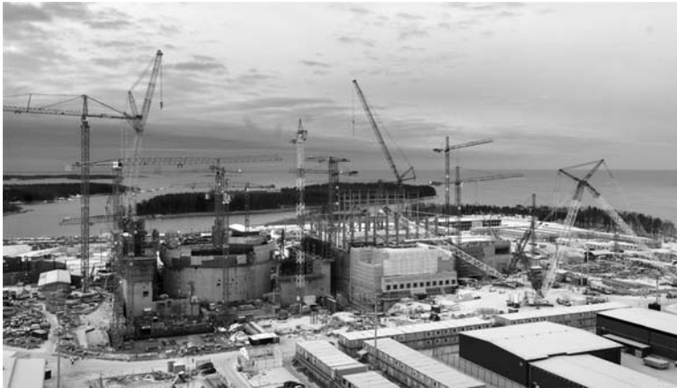
Fig. 4.14 OL3, cranes used on nuclear island – reactor building and auxiliary buildings (left) and conventional island (right) [22]
