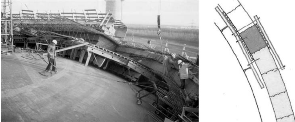
Fig. 4.17 Cupola formwork, Philippsburg nuclear power plant [17] (left), section through cupola formwork (right)
