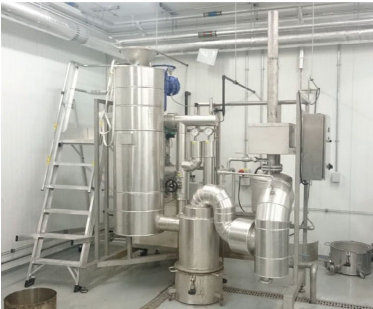
Figure 6.4 Steam explosion rig at BEACON biorefining facility (Aberystwyth University, UK). ( www.beaconwales.org )
