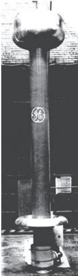
Figure 9.14 500-kV termination for the resistive cryogenic cable
