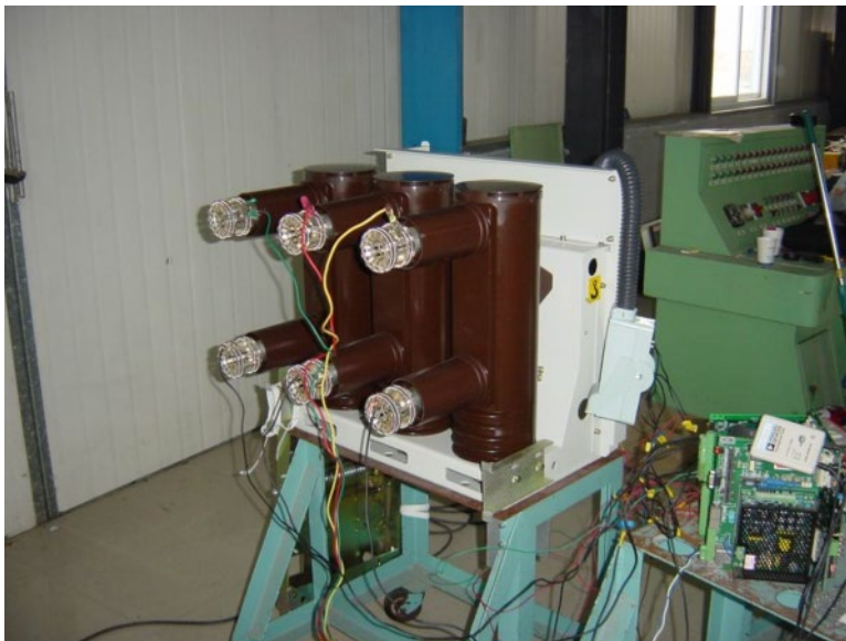
Figure 8.5 Installation and test site for on-line supervision system of breaker.
