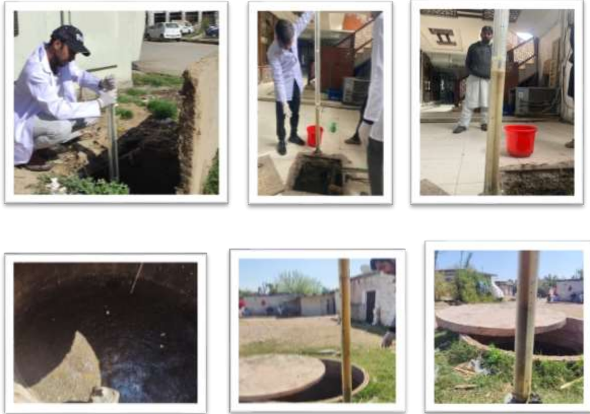
Figure 3.3 Collection of Fecal Sludge from pits and septic tanks
