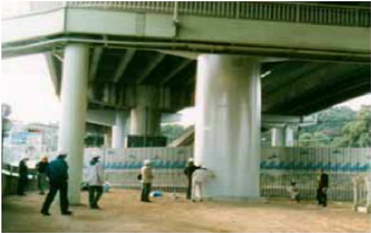
Fig. 4.6: Steel Jacket Retrofit at Hanshin Expressway in 1989, which was effective during the 1995 Kobe earthquake
