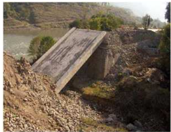
Fig 1.3 Bridges destroyed in Azad Kashmir on October 8, 2005
