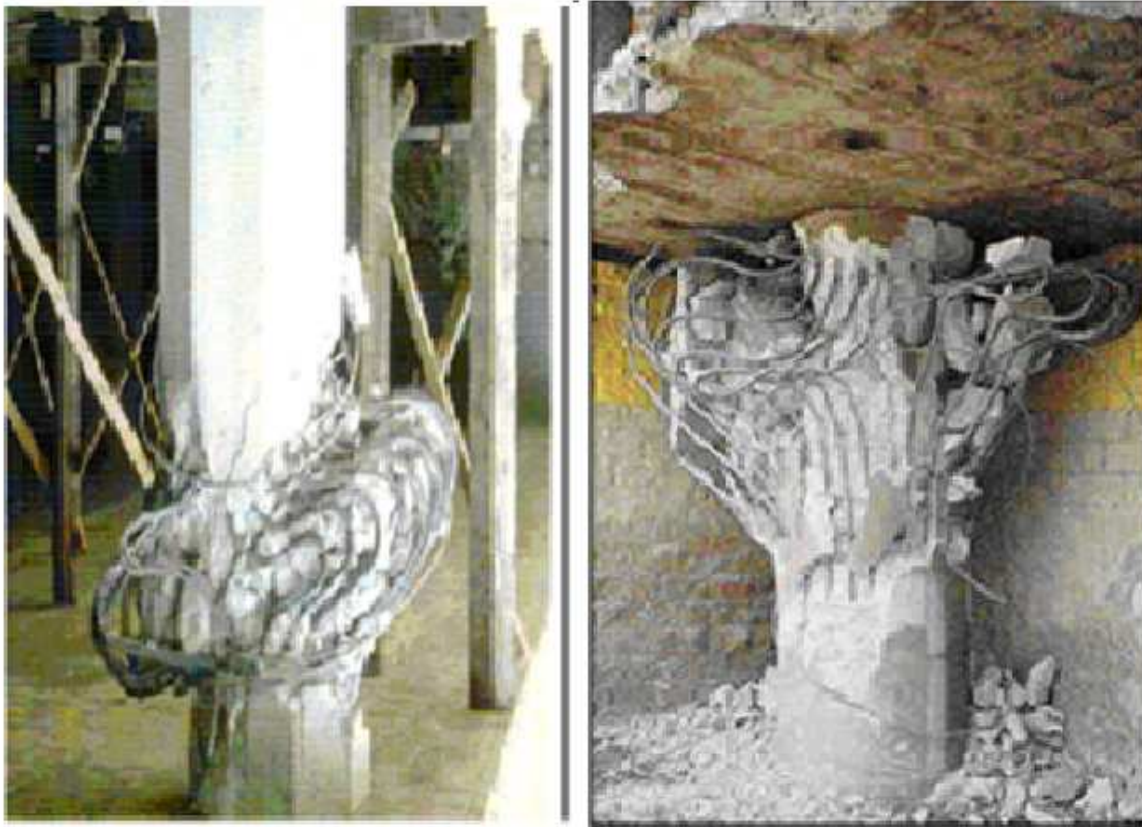
Fig 4.3: Column failures in 94' Northridge quake, (a) Spalling at column end; (b) Crushed column due to insufficient concrete-core confinement. (Cooper, et al, 1994)
