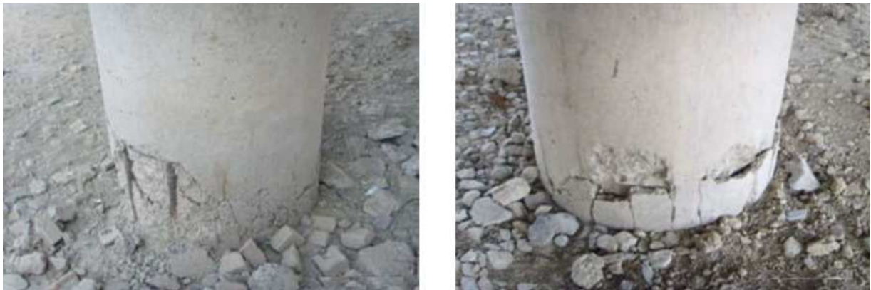
Figure 1.1: Damaged Piers of Adam Wan Bridge after October 2005 Earthquake
