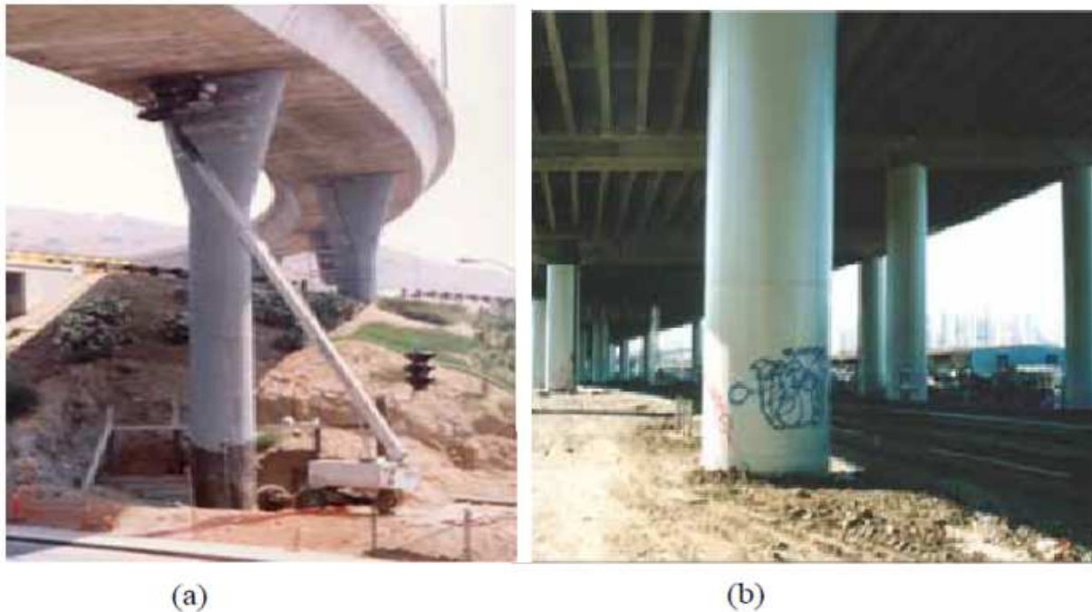
Fig 4.5: Steel jacket retrofit of columns; (a) Los Angeles, and (b) San Francisco
