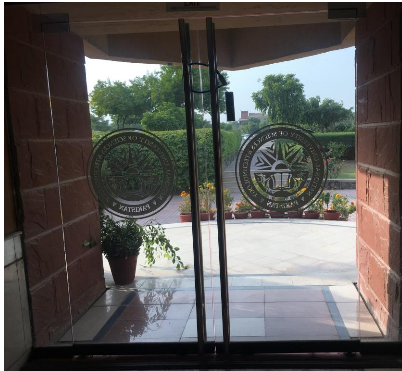
Figure 9 Glass door with gaps
