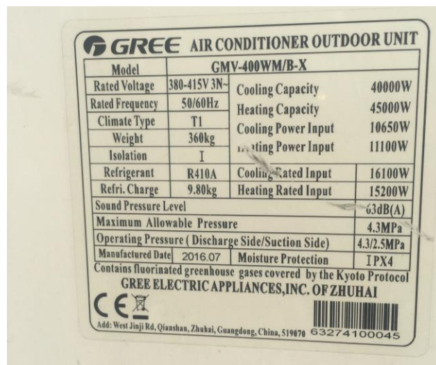
Figure 16 Nameplate of an outdoor unit installed on S3H rooftop
