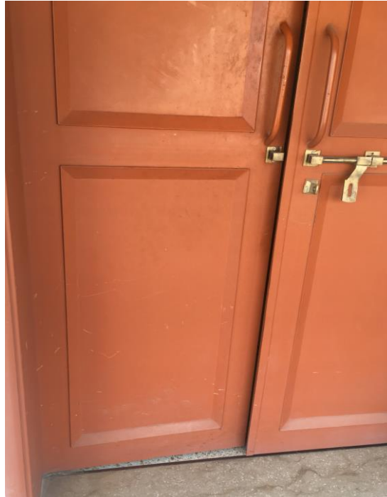
Figure 18 An example of infiltration through doors in S3H building
